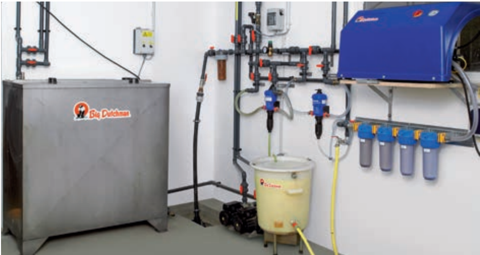
Service room with a small (60 L) and large (1000 L) stainless steel medicine mixing tank
